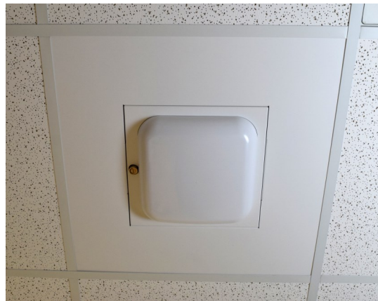
Installed in a suspended ceiling
