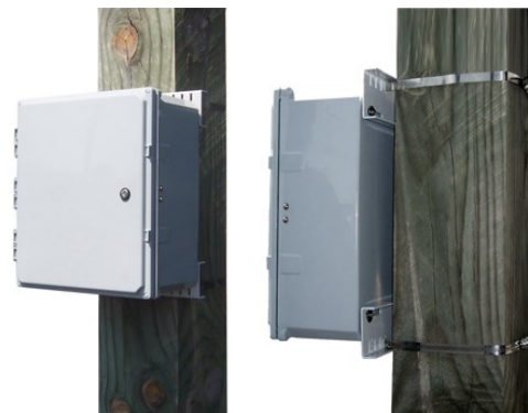
TerraWave Polycarbonate Enclosure Mounted to Large Square Wood Pole
