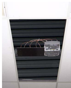
Example 3—Complete Solution Installed Above the Ceiling
