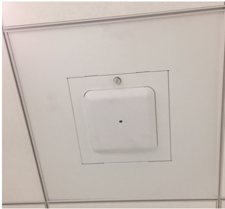
Installed in a suspended ceiling
