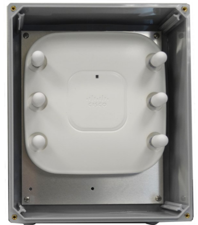
Solution with Installed Cisco 3502eAP and TerraWave Bantam Antennas
