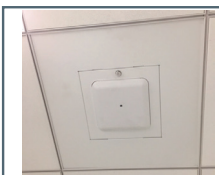
Ceiling Tile Enclosure For 335
